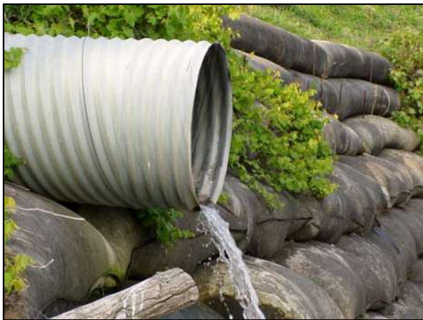
Figure 2: Storm Sewer MS4 outfall
