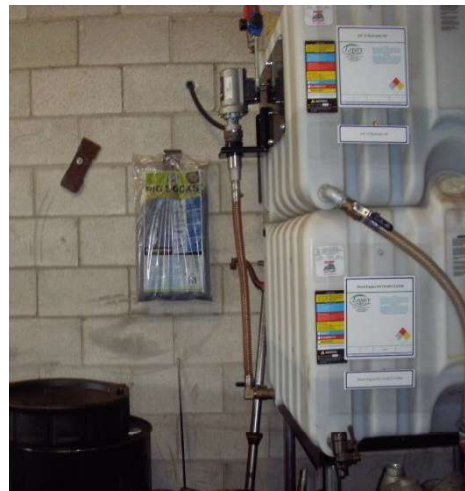
Figure 3-5. Bulk fluid loading area including sorbent material secondary
