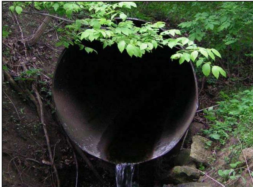
Figure 11: MS4 outfall location with illicit discharge
