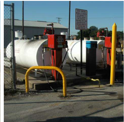
Figure 3-3. Fueling station located on pavement
